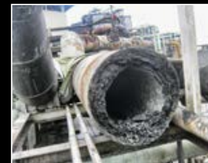
Pipe before cleaning
